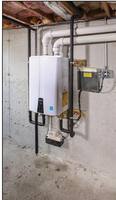
Figure 2-21: Tankless Water Heaters (Energy Saver, n.d.)
